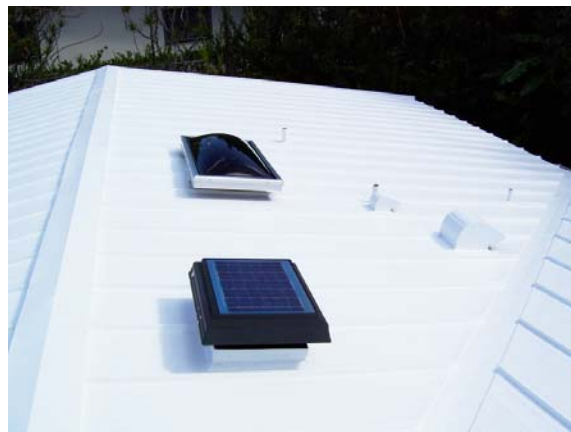
Figure 20: Skylight and solar fan
